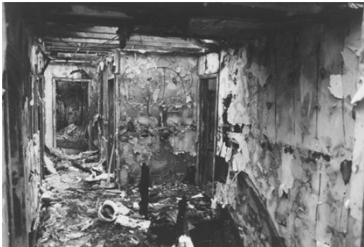
This fire started in the basement, traveled up the open stairway and killed five students on the second floor of this fraternity. ©NFPA 2001 Used with permission
